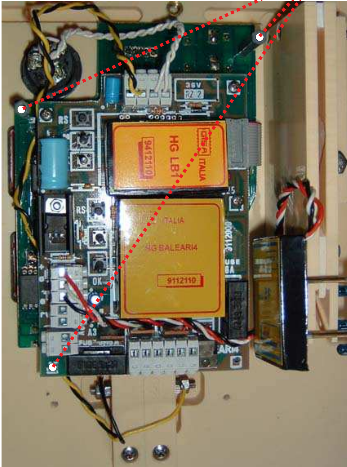
Mod. BALEARI4 (inside the board)
